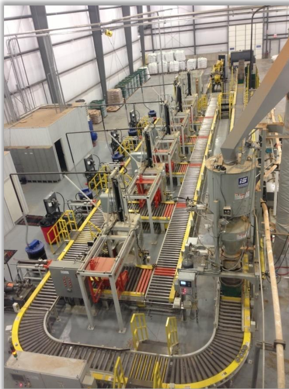
Automated Tub Press System
